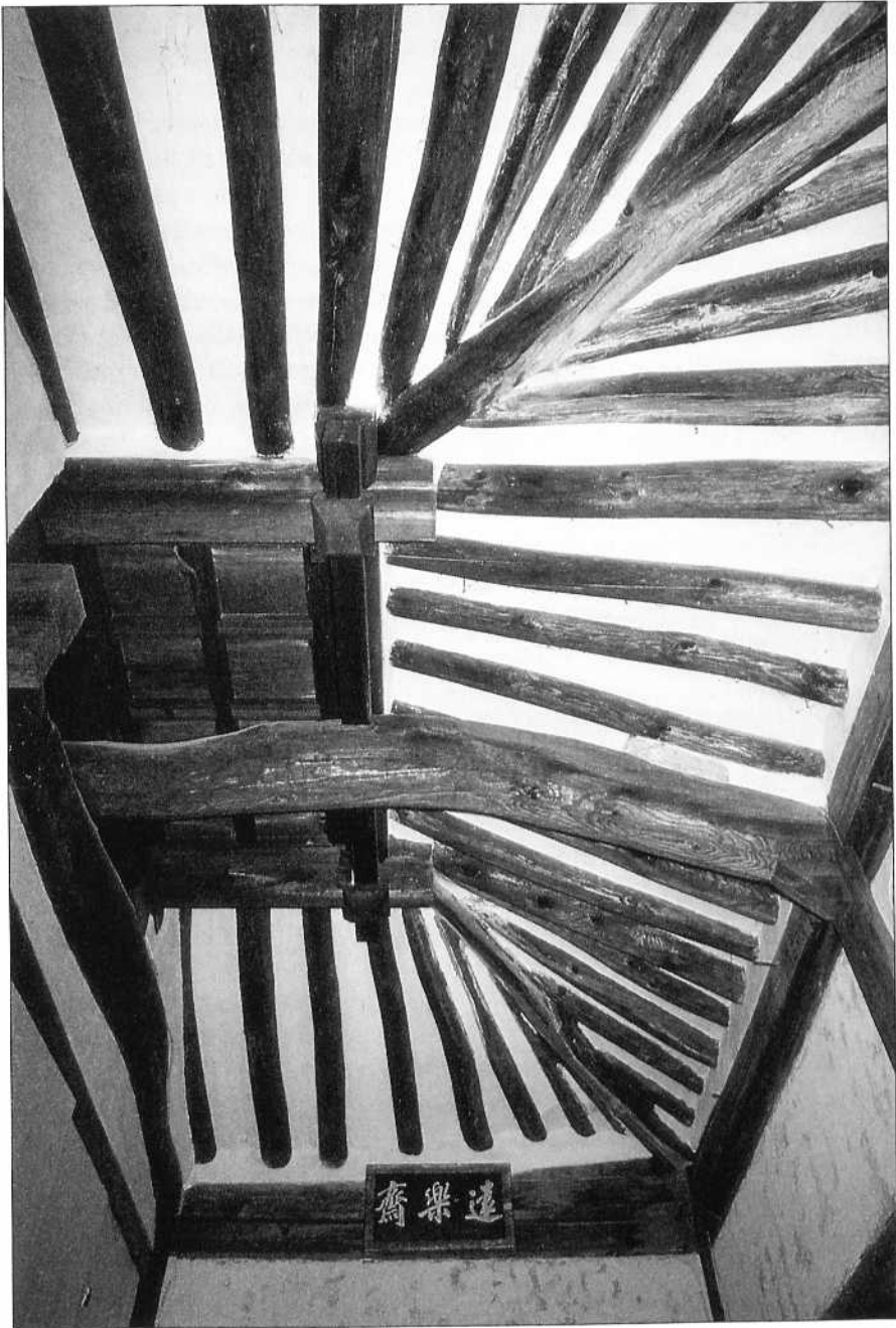
Ceiling in the former country house of a Korean aristocrat. Typical of traditional Korean residential architecture, there are no ceiling boards and the wooden roof beams are visible. In Japan, this kind of ceiling, termed funazoko-gata (ship's-bottom style), is sometimes seen in rustic tearooms.
